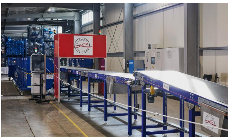
Figure 16 : Looper Textile automated sorting line in Polch, Germany
